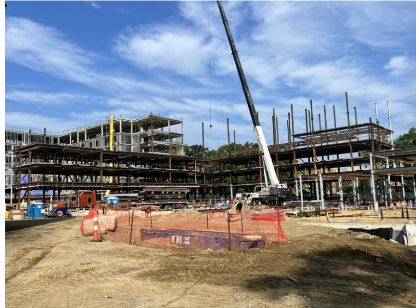
View looking northeast of steel construction on one of two L-shaped wings of the Residence Hall
