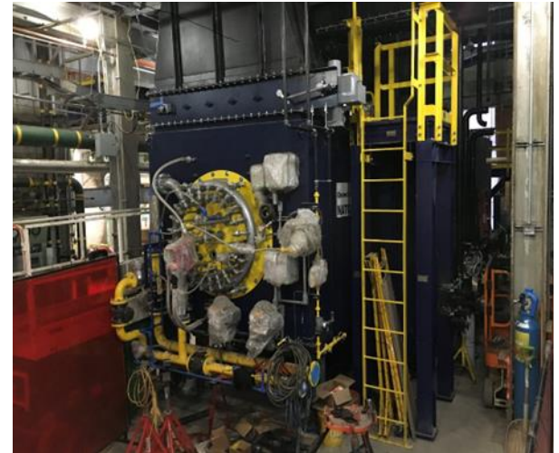
New Packaged Boiler installed in the Central Utility Plant
