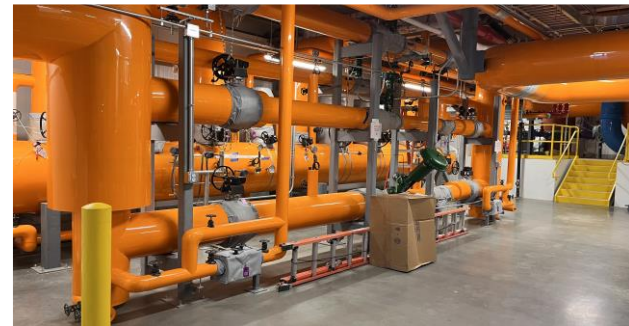
SUP Interior View of 125 psi Steam Header
